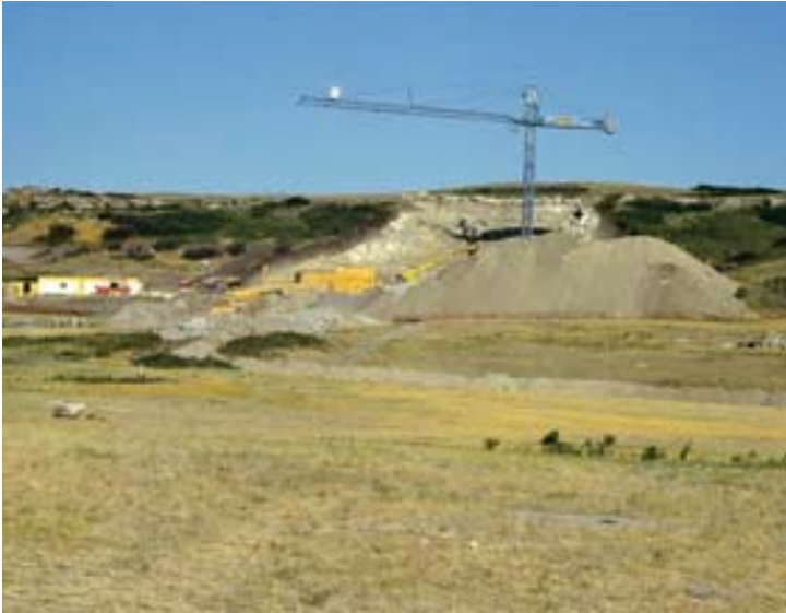
Building the Head-Smashed-In Interpretive Centre required blasting a huge hole in the bedrock to situate the seven-storey building. (Courtesy Royal Alberta Museum)
